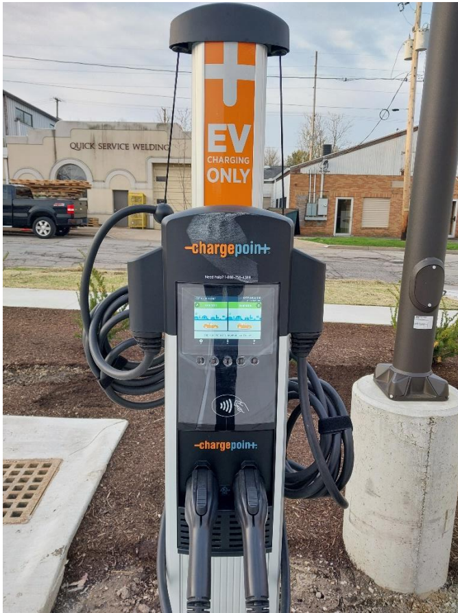
Kent City Hall EV Charging Station South-Side operating screen
