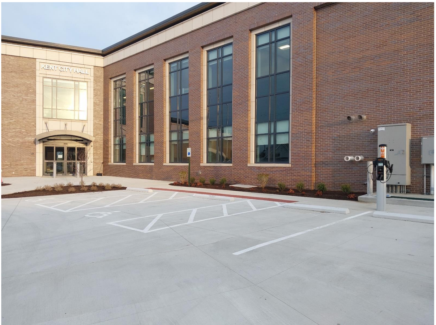
Kent City Hall EV Charging Station North-Side
